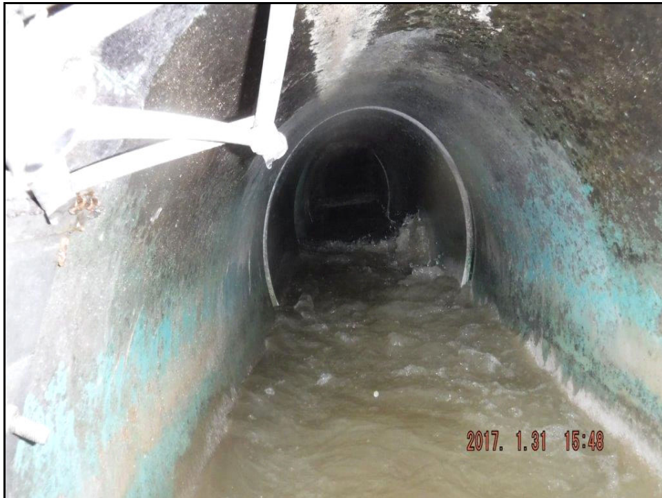
North Inflow Pipe
