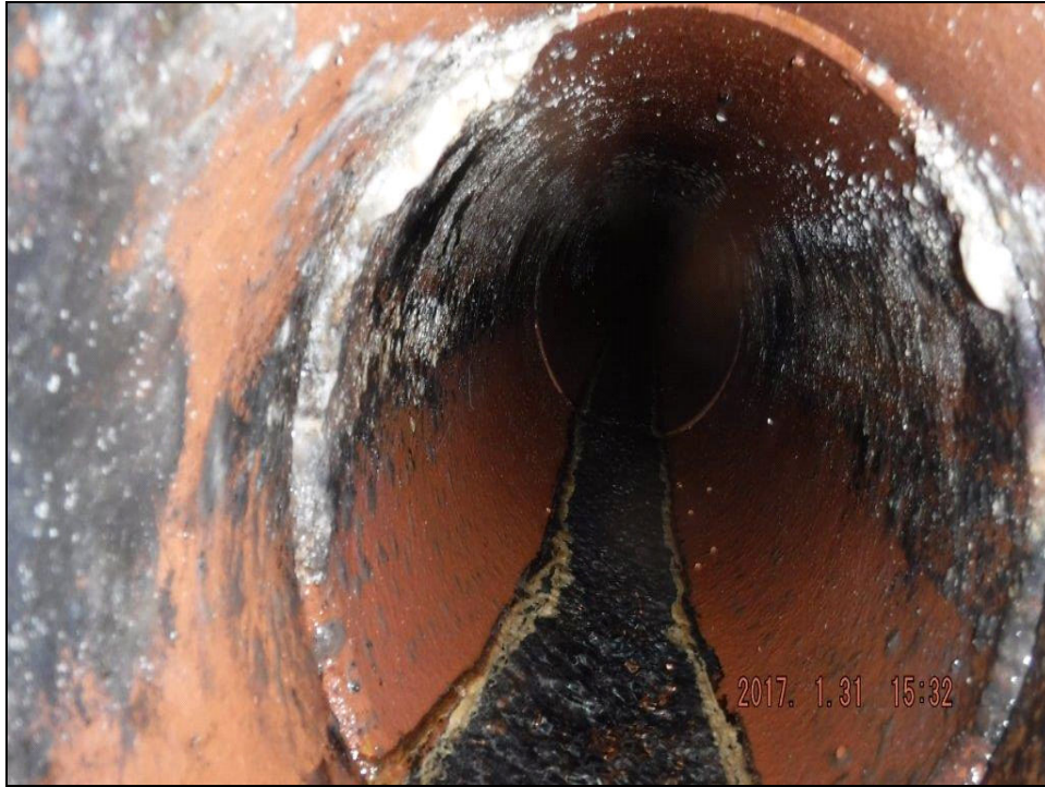
East Influent Pipe
