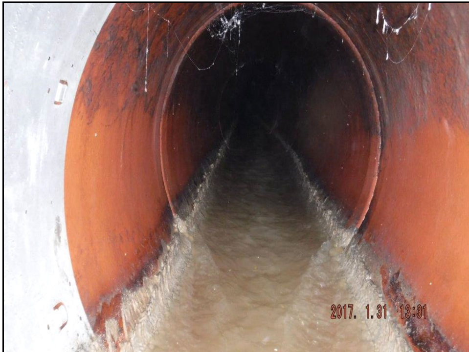
East Influent Pipe
