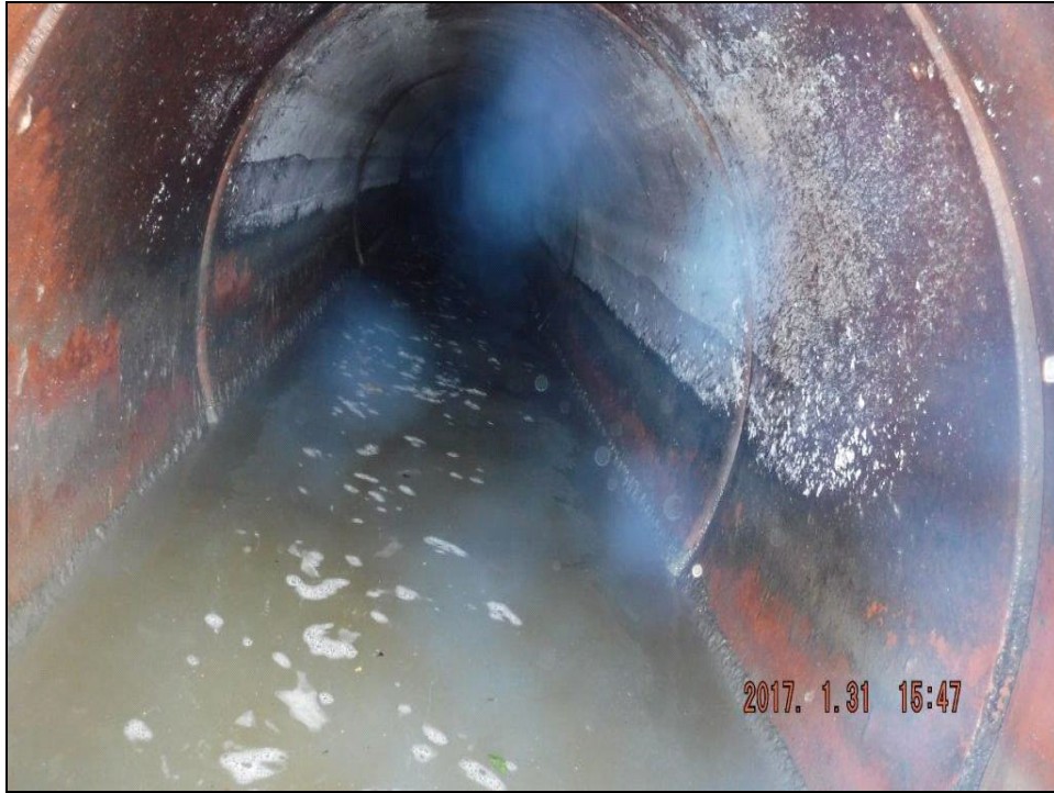
West Influent Pipe
