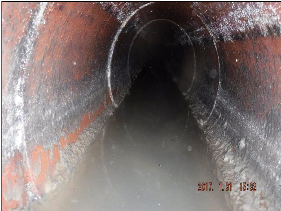
North Influent Pipe
